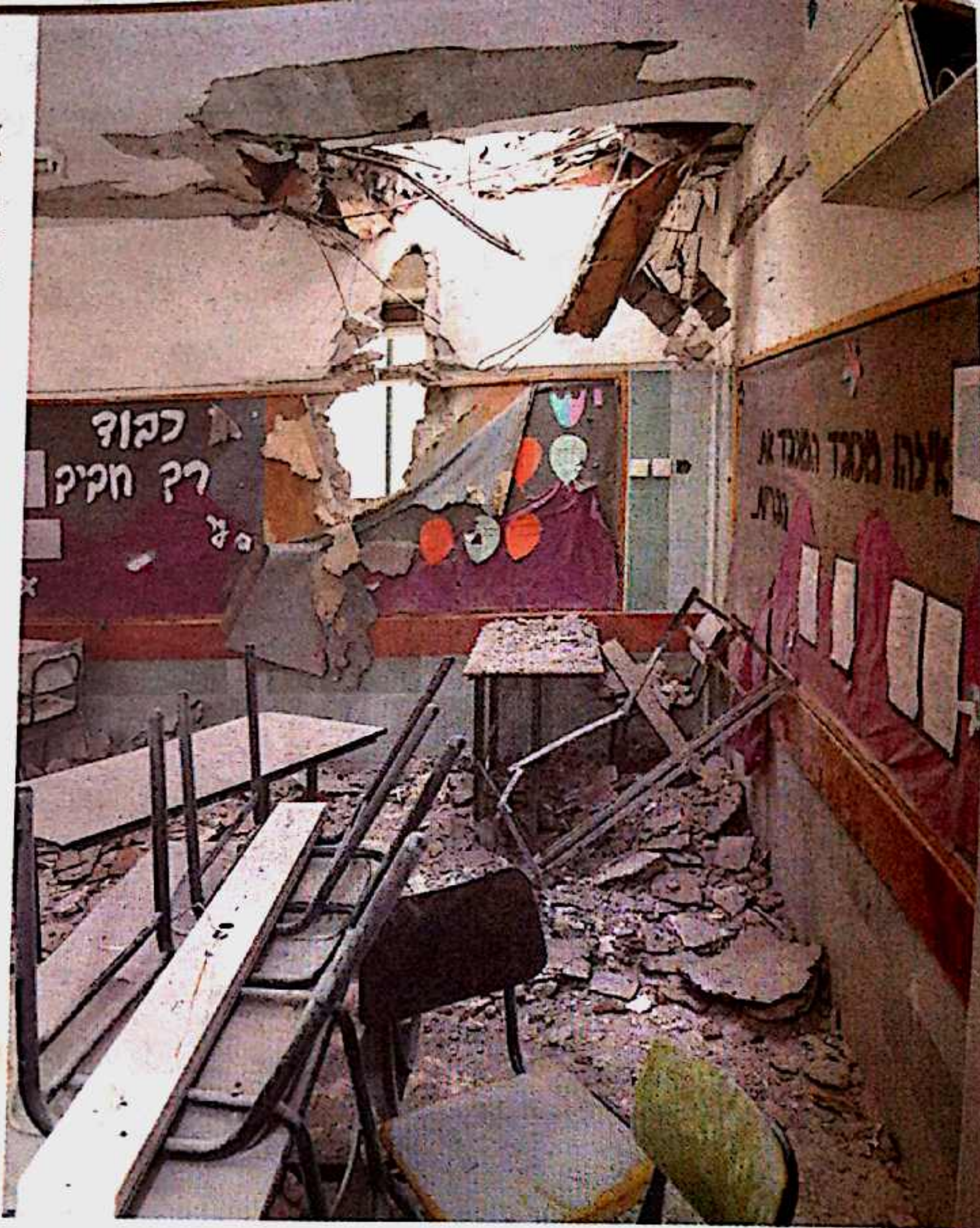
AFTERMATH OF rocket damage in an elementary school classroom.
